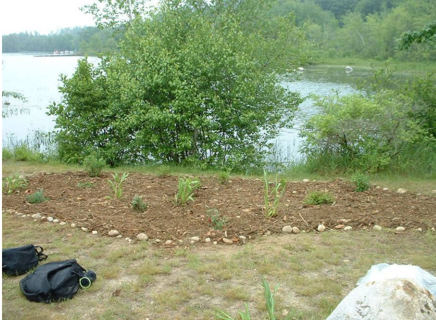
The installation of this landscaped buffer is in progress. Note how the design enhances, not blocks, lake views.
